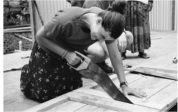
Even at work on the construction site, Elizabeth Randazzese '00 honored the custom of the Fiji women by wearing a modest top and skirt.
