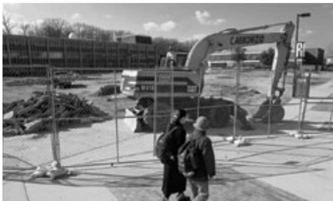
Excavation for the new science building began this spring semester, making Meditation Walk an ironically busy, noisy passage through the north side of campus. Construction will produce a spectacular facility designed for and dedicated to studies in biology, chemistry and physics.
